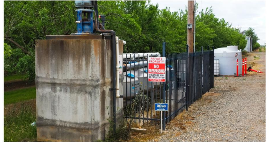
Filtration System | Arboleda 77
