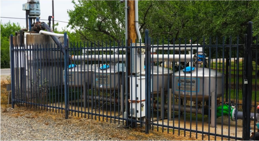
Filtration System | Arboleda 77
